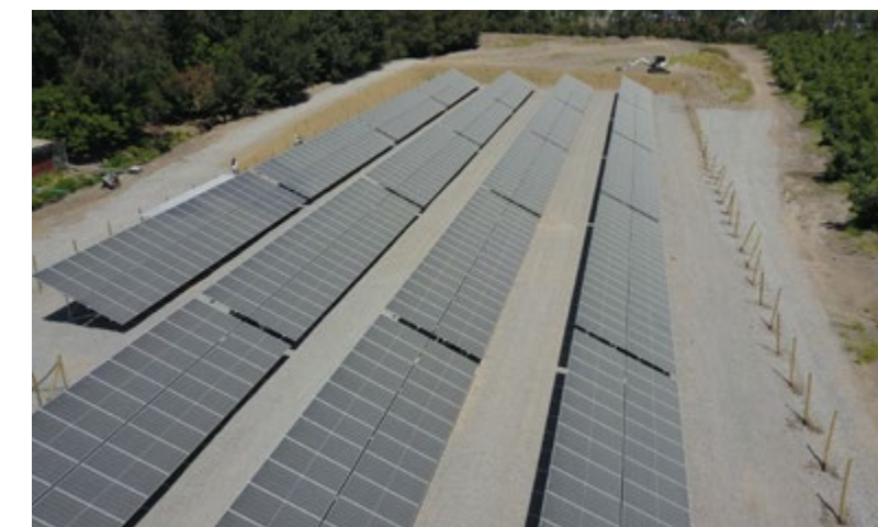
Photovoltaic system Corporate Building
