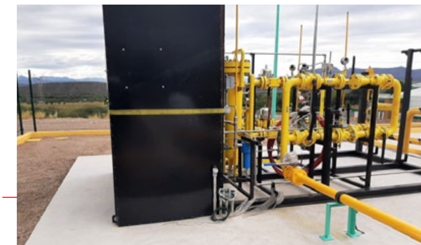
Replacing fuel at Molymex (Liquefied petroleum gas for natural gas)
